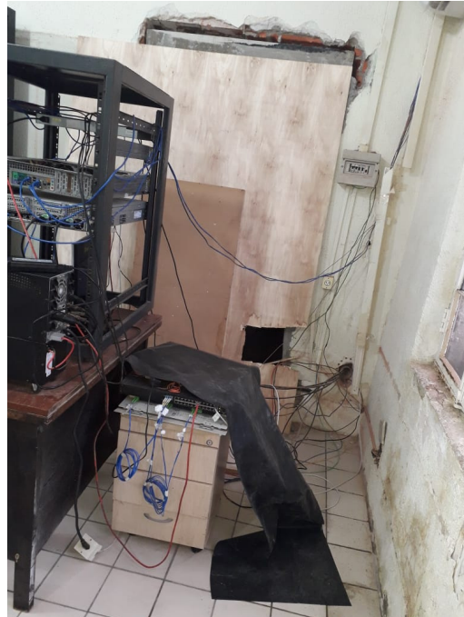
Figura 5 – Switch principal do CPD
